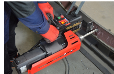
Out of position drilling
